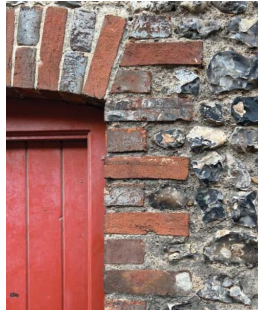
Examples of brick and flint including cobbles and brick used in pathways.
